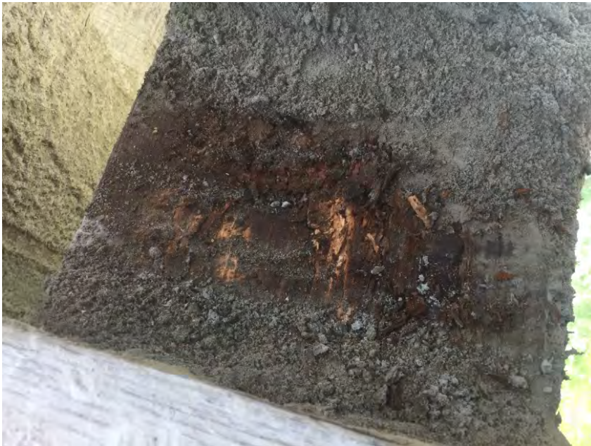
Random tie exposed with signs of decay
