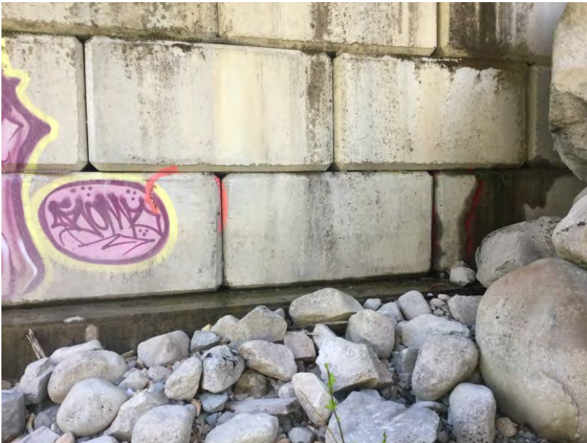
Surficial cracking of lock blocks at right bank
