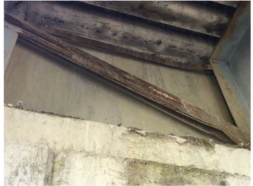
End diaphragm at right abutment heavily corroded
