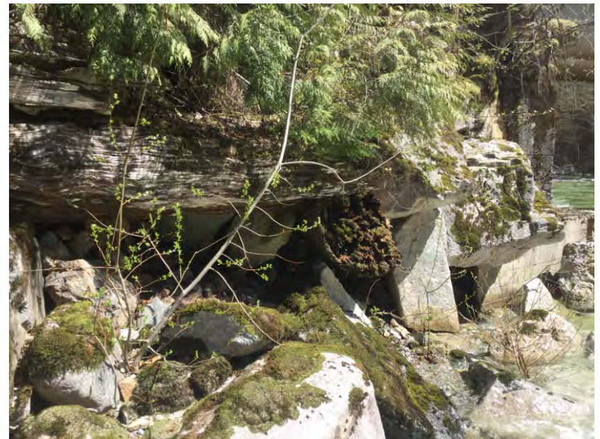
Logs buried in fill at left abutment behind CIP
