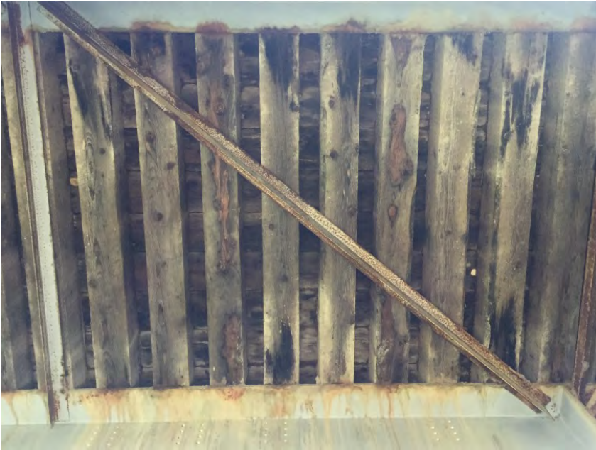
Indications of deck rot throughout
