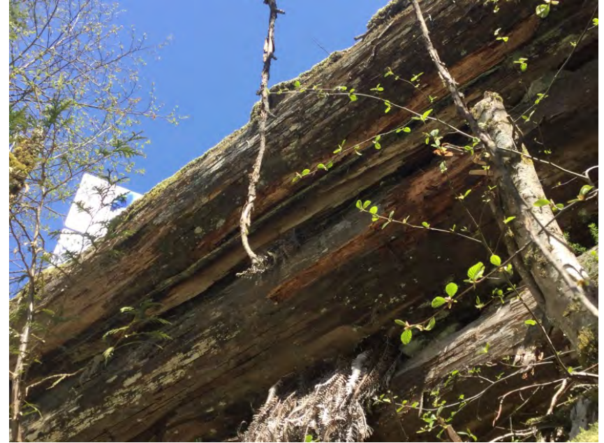
Up to 50mm sap rot on log wingwall on left bank
