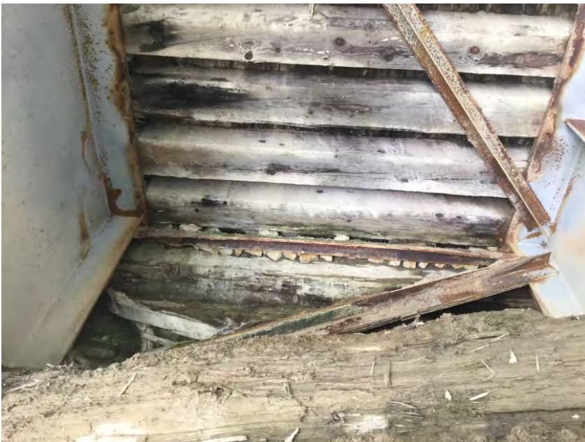
Bracing at left bank appears heavily corroded
