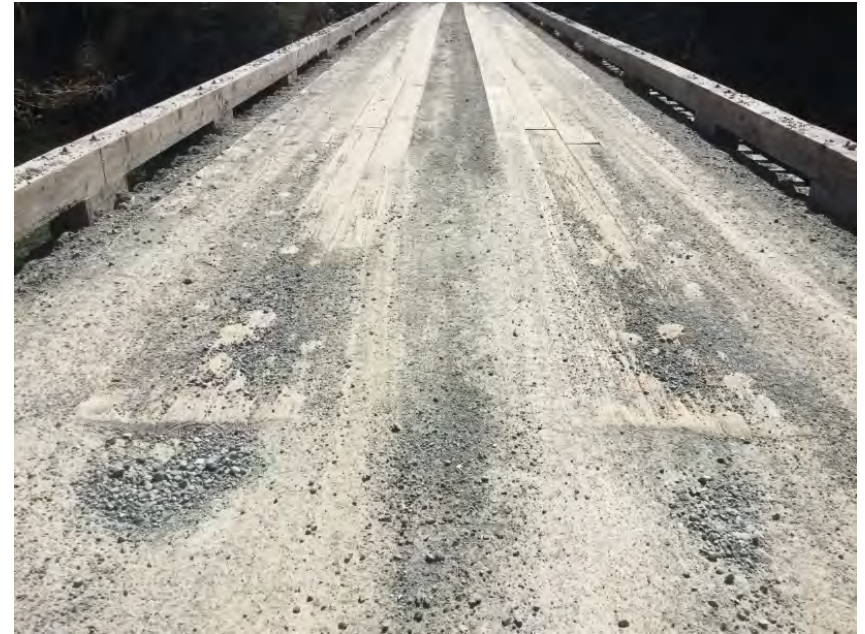
Deck - wearing on wheel path at both approaches
